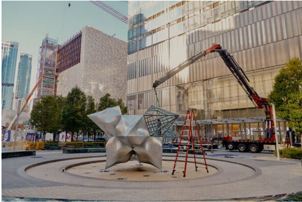
A construction crew installing Frank Stella's sculpture "Jasper's Split Star" in front of 7 World Trade Center. Credit: Vincent Tullo for The New York Times
